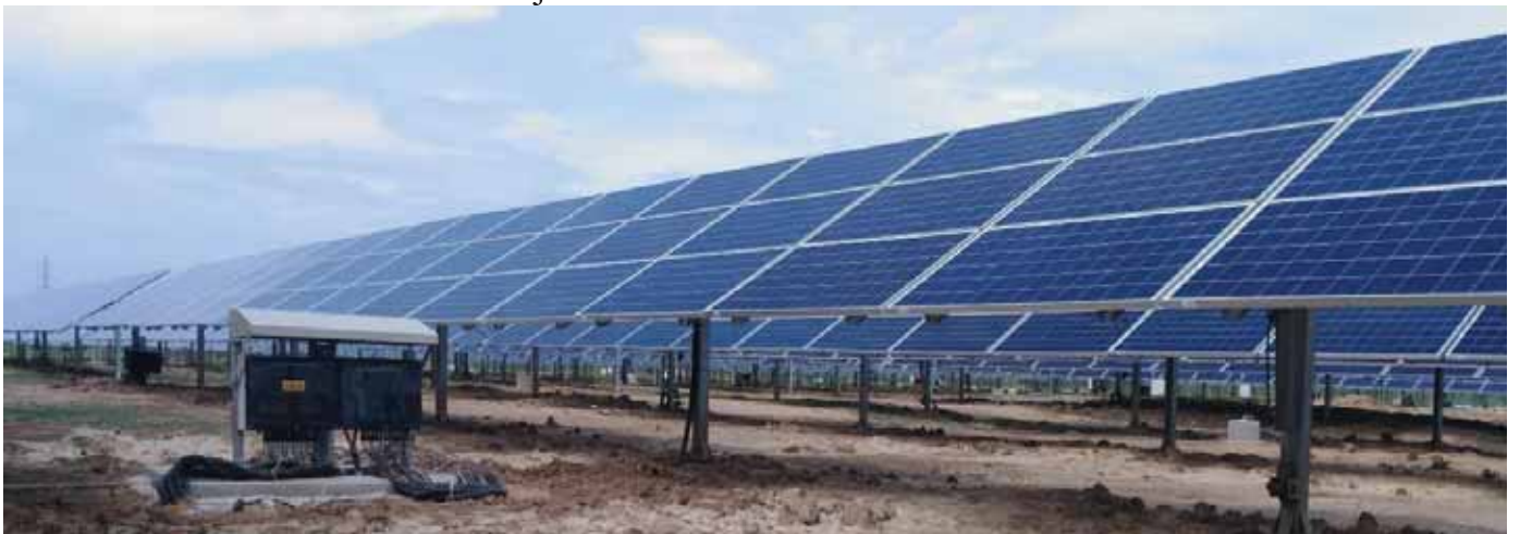
20 MW (Megawatts) in Vengappally, Telangana, India (The Highest Capacity of the Power Plant Executed in a Single Project)
