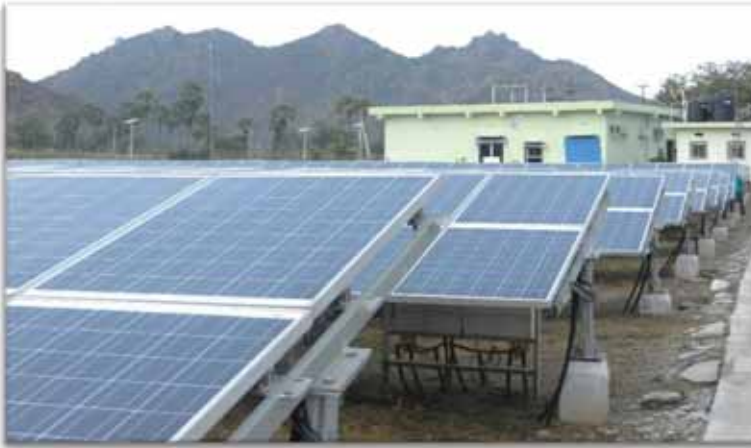
2 MEGAWATTS - GUNDUR, ANDRAPRADESH, INDIA
