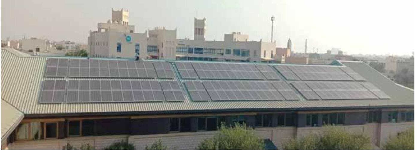
Middle East Project Executed : 1.25 Megawatts (MWp) in the Kingdom of Bahrain for M/S Techmaaxx Projects & Services WLL -Bahrain for a School at Saar.
